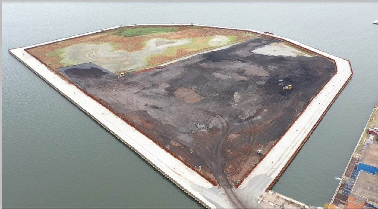
Aerial view of the geogrid and geotextile being layered over secondary materials.
