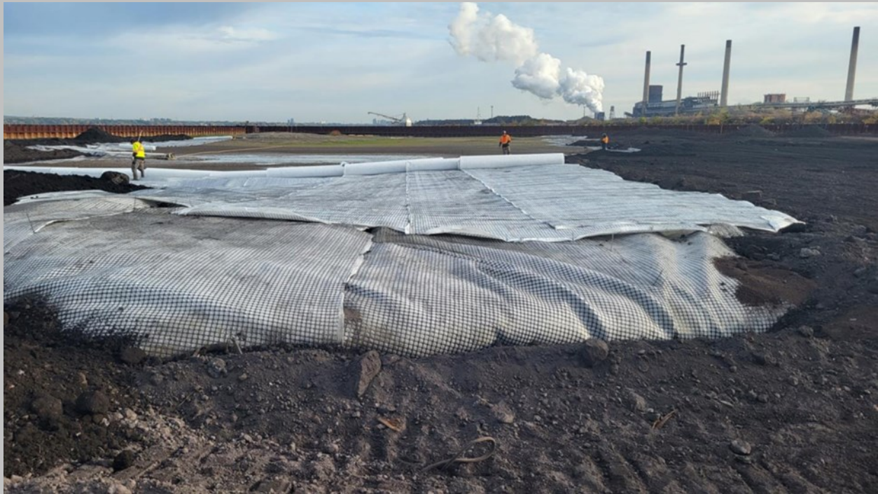
Surface view of the geogrid and geotextile being layered over secondary materials.
